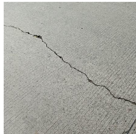
Fig. 2. Cracked Road Image
