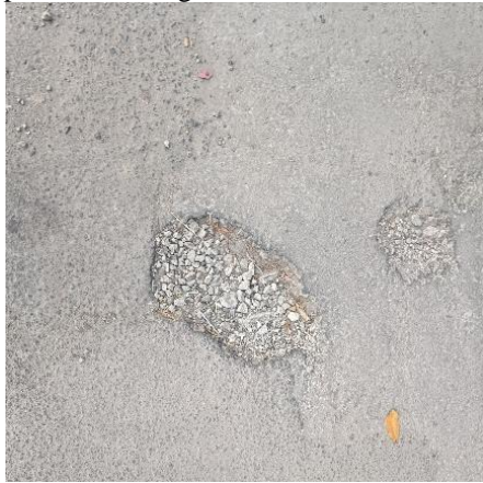
Fig. 3. Pothole Road Image
